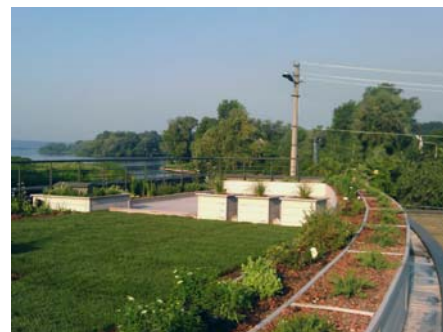
Shortly after the application of the turf rolls and the planting of the single planters.
