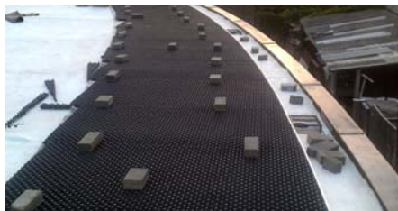
The drainage element Floradrain® FD 40-E has been applied on the entire area; the Filter Sheet and the System Substrate respectively the decking with planters have been applied on top.
