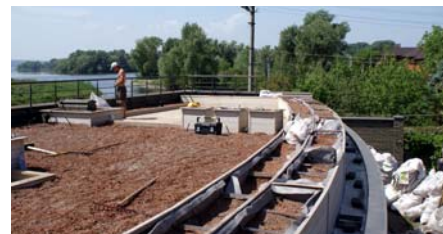
The System Substrate has been transported onto the roof by means of BigBags.
